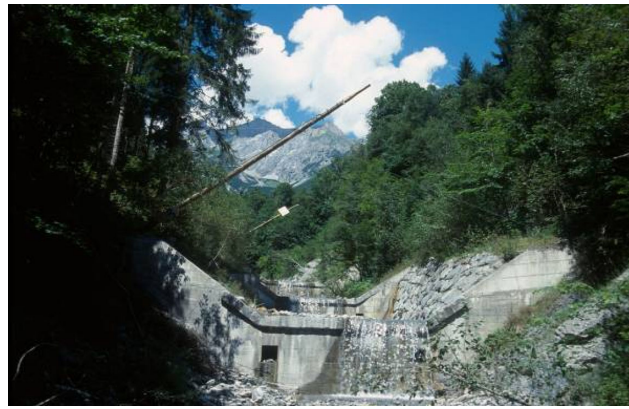
Figure 4. Flow depth sensors installed over a series of check dams at the monitoring station Grins (middle reach).
